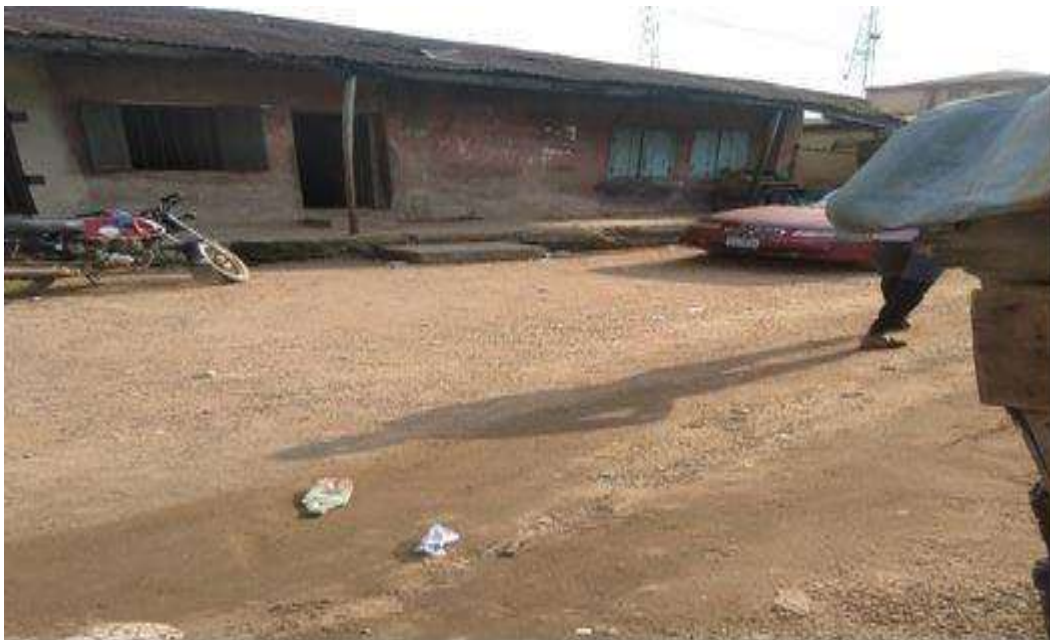
Figure 12. Picture showing the bad condition of the house. Source: Author's Fieldwork, 2021.
